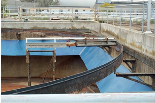
Density Current Baffles
